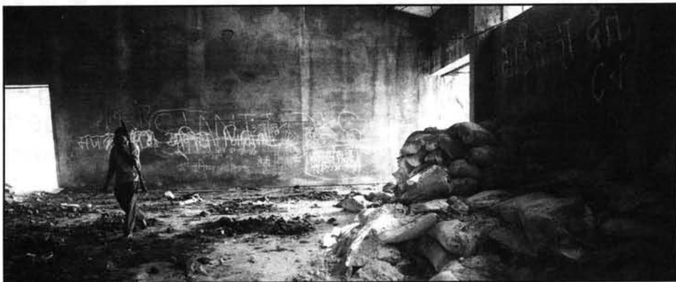
THE remains of the chemicals still lie scattered on the factory floor
